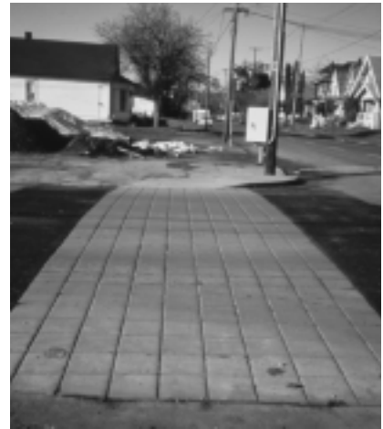
A change in paving materials at pedestrian crossings can make the crossing more visible.
