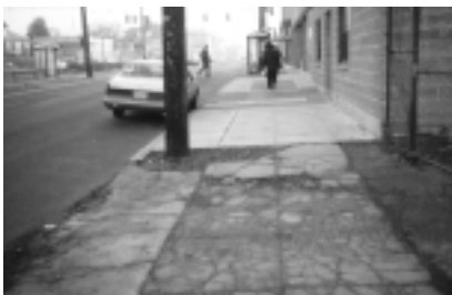
Some of the older sidewalk on Alberta Street is in disrepair.
